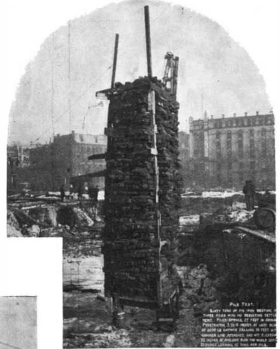
TEST OF PILES—60 TONS OF PIG IRON ON THREE PILES; NO SETTLEMENT.
