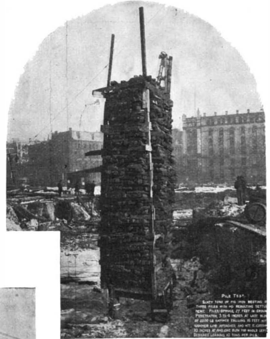
TEST OF PILES—60 TONS OF PIG IRON ON THREE PILES; NO SETTLEMENT.
