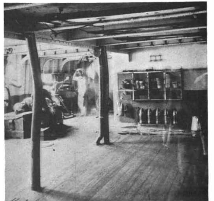
5.—Stanchions Bent by Blast of 12-inch Gun on Deck Above.
