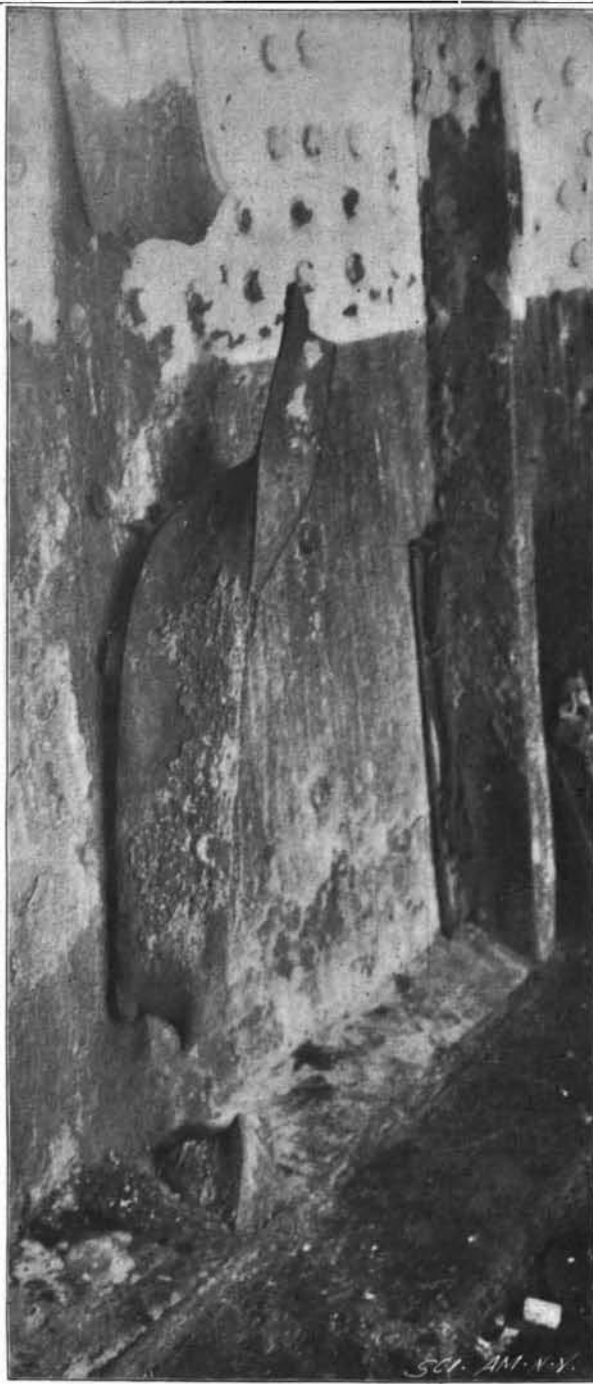
7.—Starboard Ship's Frame on Gun Deck Cut in Two Places by Fragments of 6-inch Shell.
