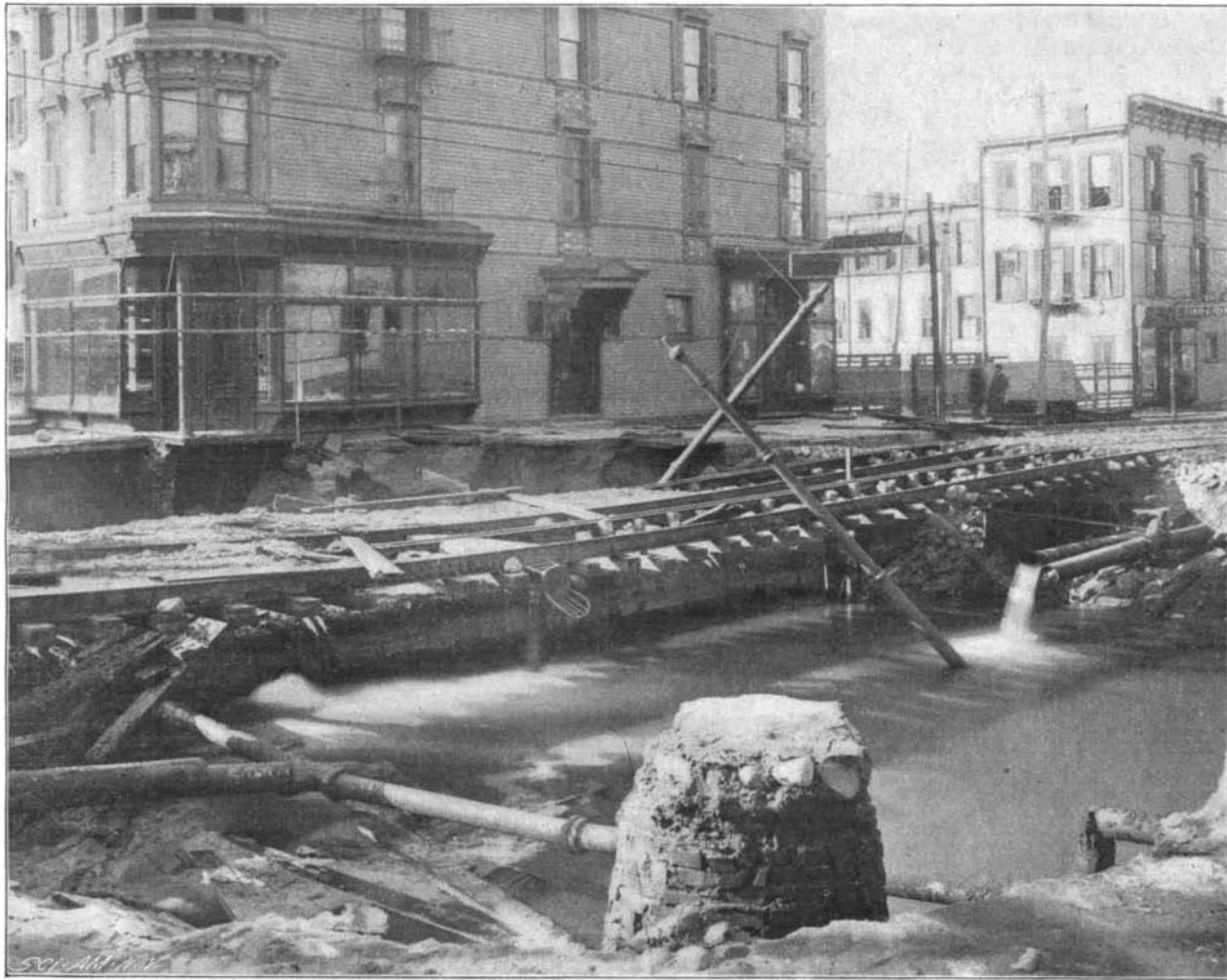
BREAK IN A 48-INCH WATER MAIN IN BROOKLYN, N. Y.
