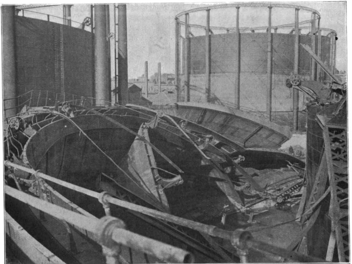
3.—LOOKING DOWN UPON THE WRECK OF THE TANK AND THREE LOWER SECTIONS OF THE HOLDER.
