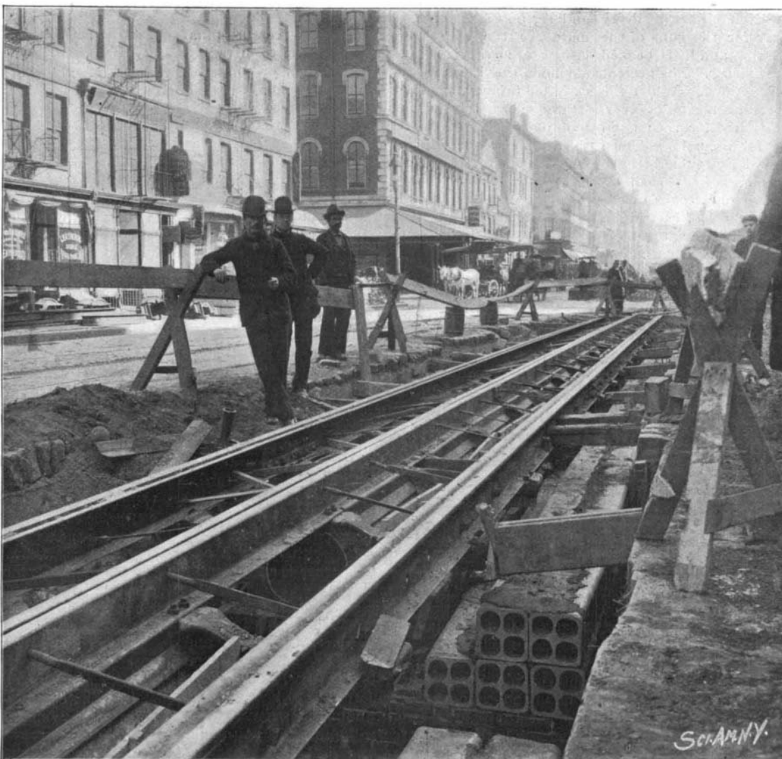
2.—CONSTRUCTION OF NEW UNDERGROUND TROLLEY ROAD ON CANAL STREET, NEW YORK CITY.
