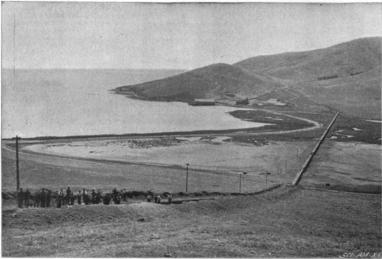
PIPE-LINE ACROSS MARSH, CARRIED ON TRESTLES.
