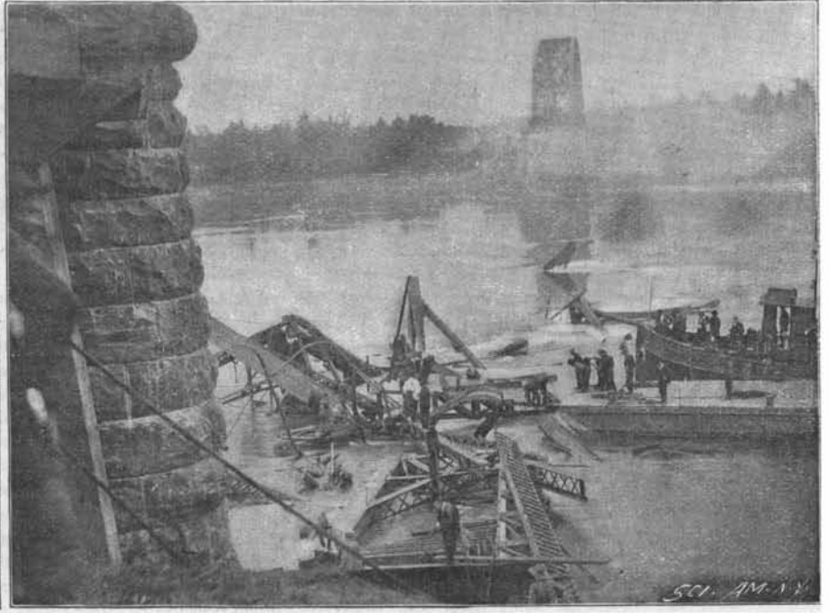
WRECKAGE OF THE SHORE SPAN AND FALSEWORK.
