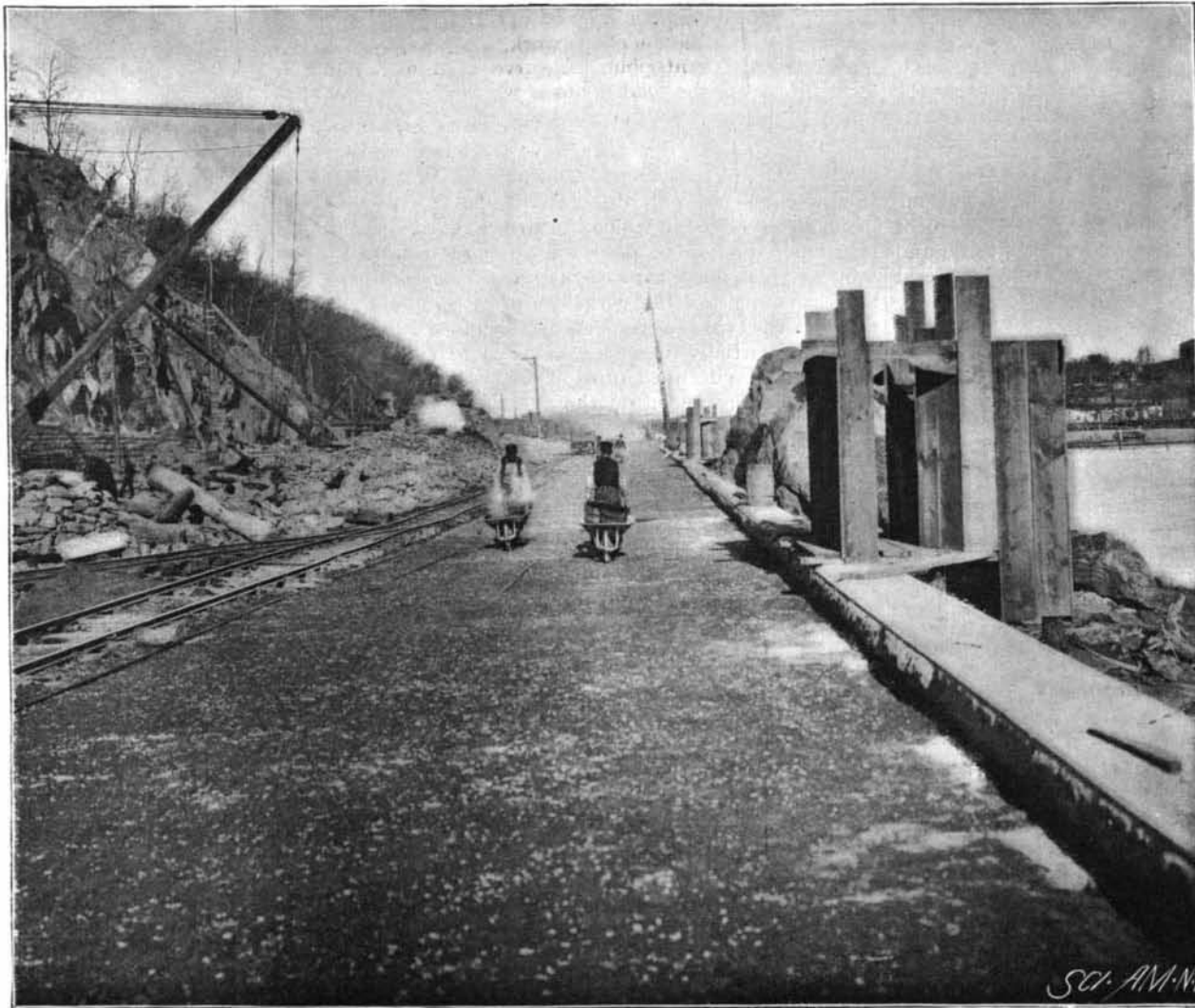
THE HARLEM RIVER SPEEDWAY—LAYING CONCRETE FOUNDATION FOR ASPHALT ON THE EASTERLY SIDEWALK.
