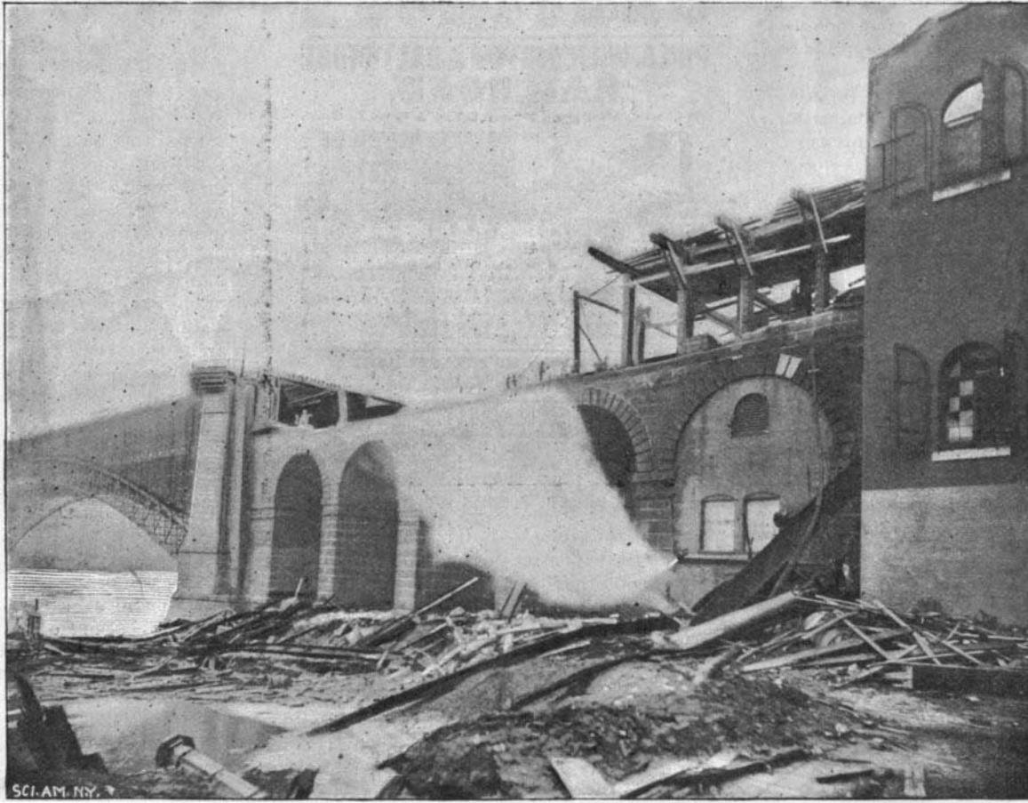
THE ST. LOUIS BRIDGE AFTER THE GREAT STORM OF MAY 27, SHOWING INJURY TO STONE WORK ONLY.
