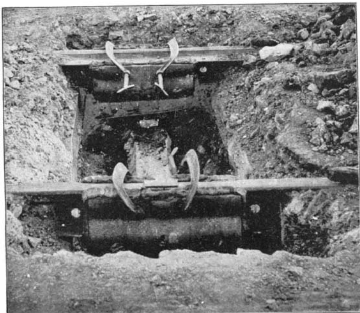
MOULDS ON JOINTS.
