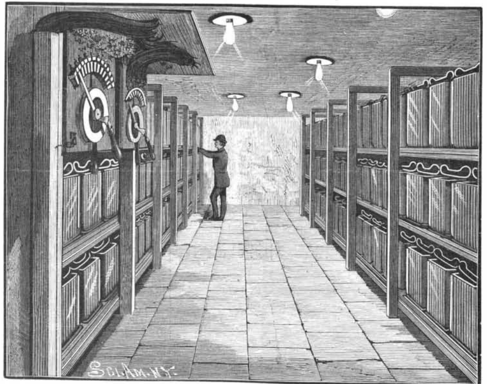
STORAGE BATTERY ROOM.
