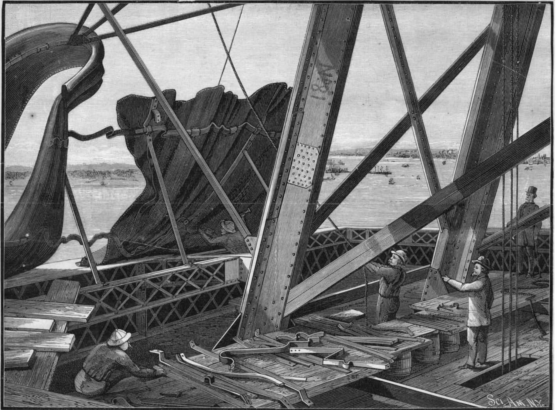
STATUE OF LIBERTY.—VIEW AT TOP OF PEDESTAL, SHOWING THE SHELL AND BRACING.
