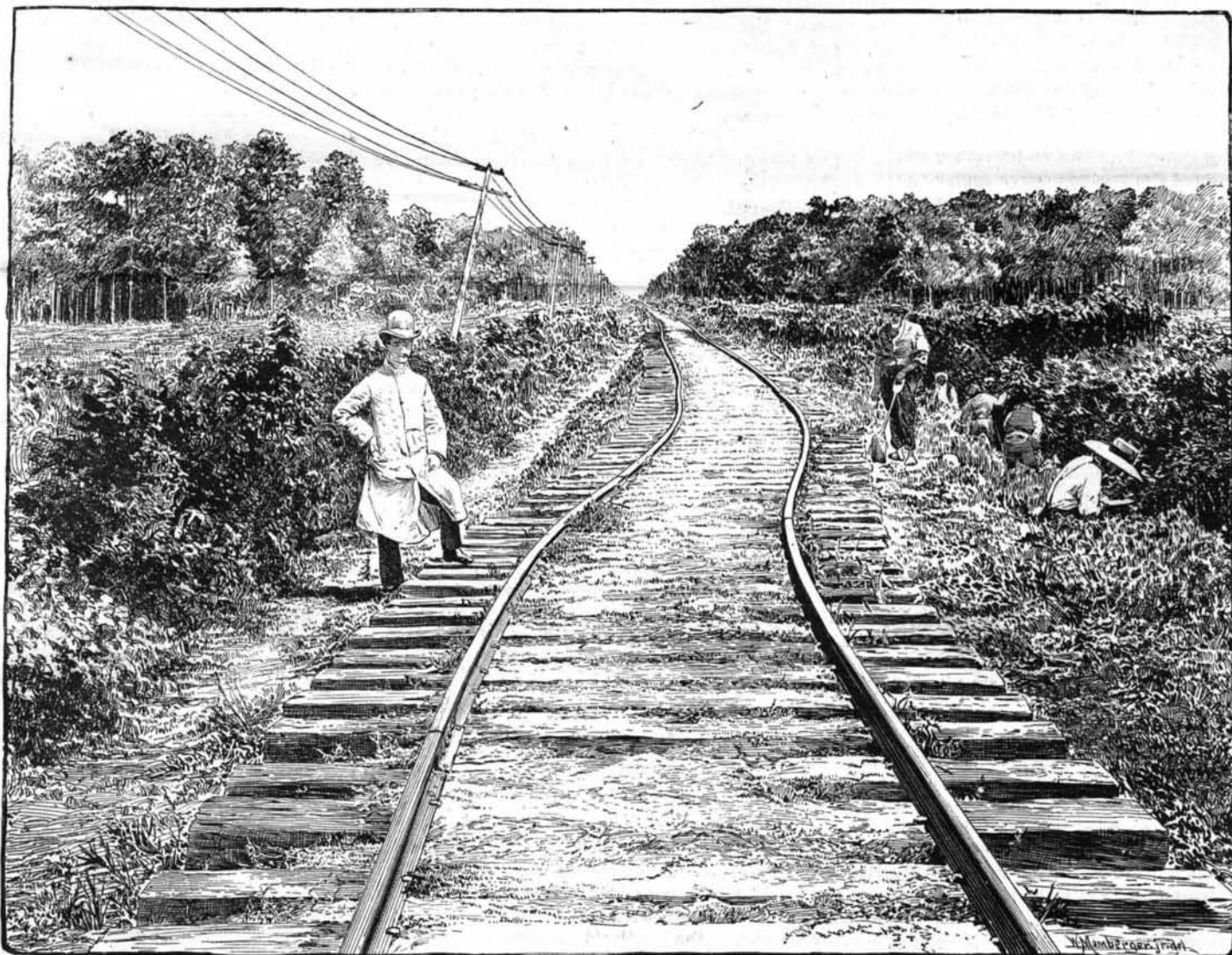
THE SOUTH CAROLINA RAILWAY.—VIEW NEAR TEN MILE HILL AFTER THE EARTHQUAKE OF AUG. 31, 1886.
