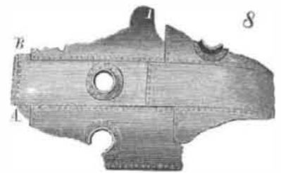
Girdle of plates torn from No. 2 boiler. A B, line of initial rupture. I, locality of leak mentioned by the engineer.
