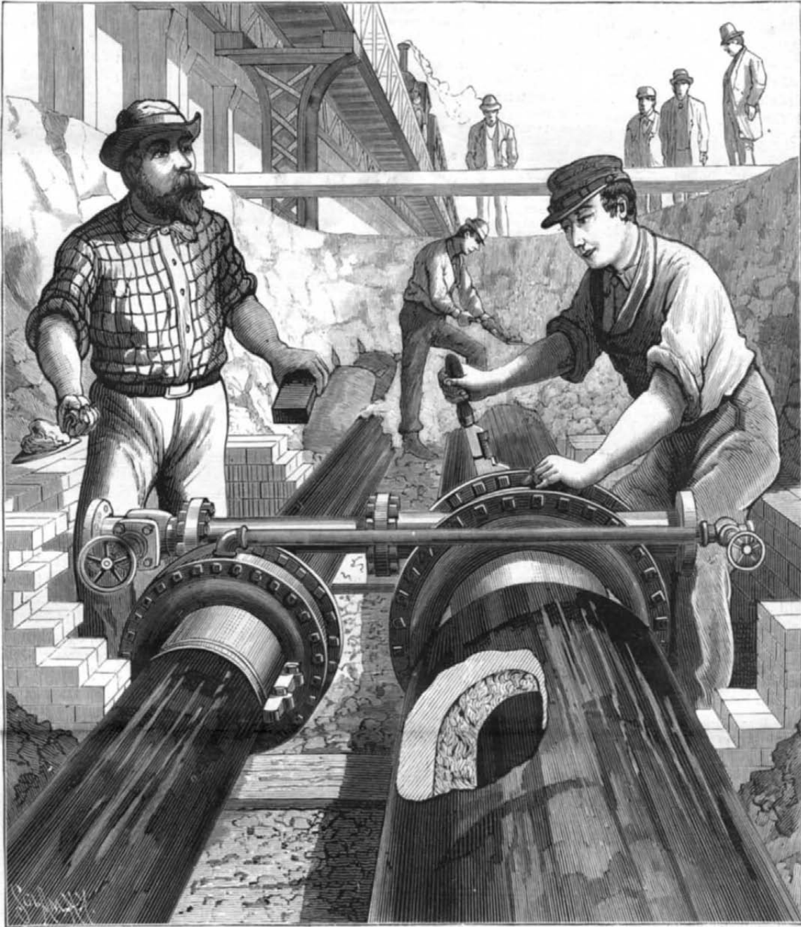
STEAM DISTRIBUTION—THE STEAM PIPES AND EXPANSION JOINTS.
