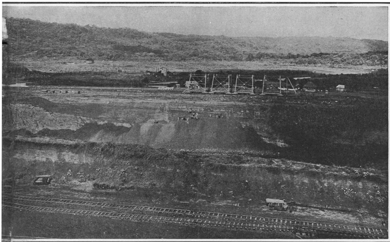
Between and running from right to left is the excavation for the locks, which will be 380 feet wide and 3,800 feet long. They will consist of a huge monolithic concrete structure. The concrete mixers in electrically-operated cars, picked up by the cableway, and deposited in place.
