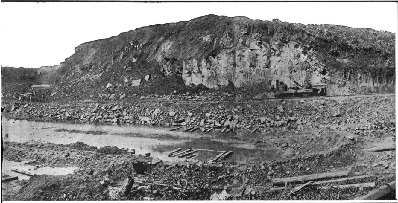
The spillway. The above photograph is taken looking through the completed spillway excavation, which will be lined with a heavy covering of concrete commenced and is now well under way.
