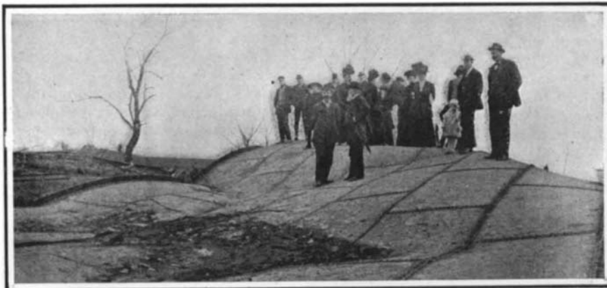
Side of one of the tanks which was found over 100 feet from its foundation.
