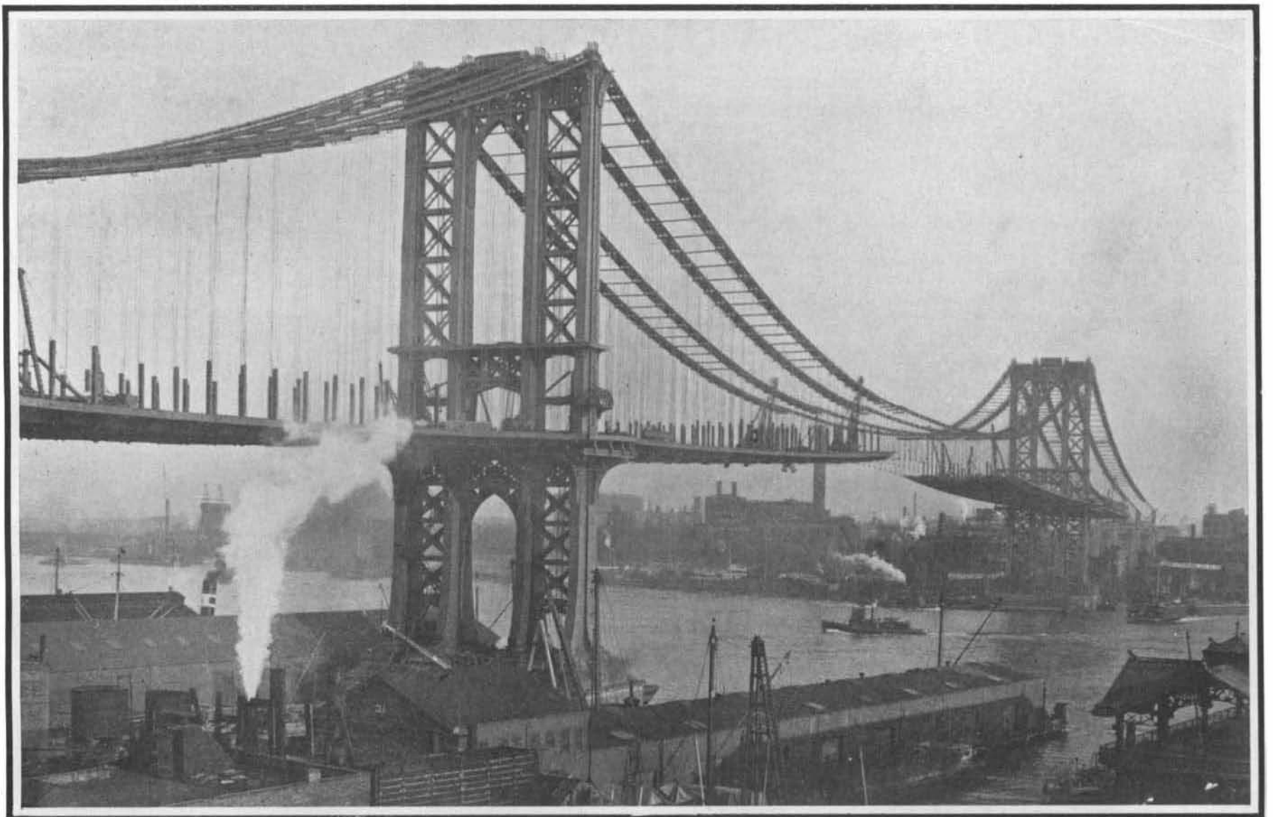
The upward curve of the completed roadway is due to the partial loading of the cables, which are depressed near the towers and raised at the center. When the floor is completed it will lie in a true curve.
