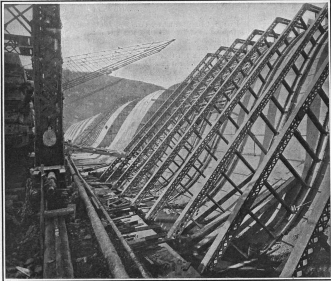
View showing the steel forms used in molding the face of the dam.
